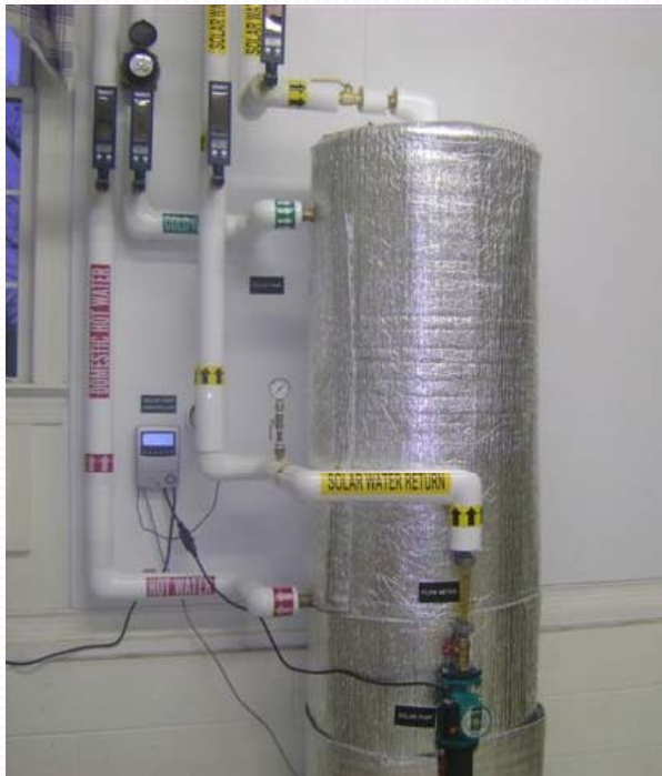
Solar Thermal Drain Back Tank & Piping
